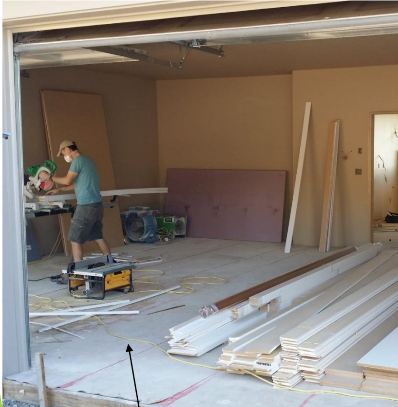
Millwork carpenter cutting in the garage to keep dust out of the house
