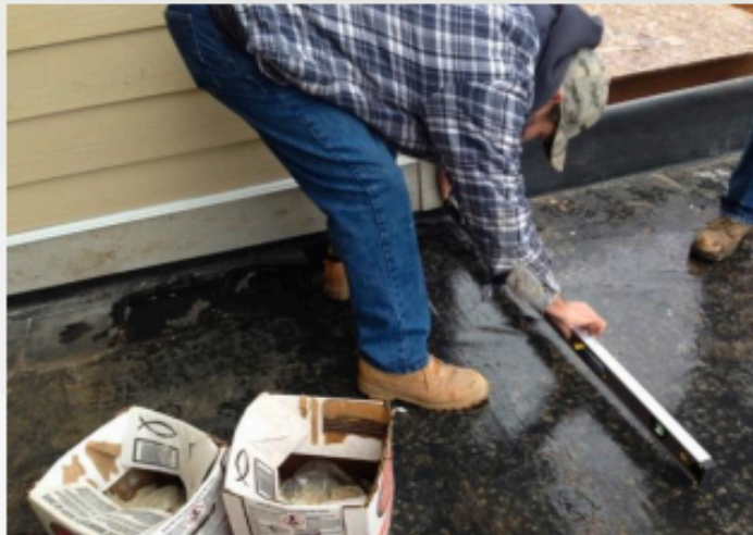
Left: Carefully checking level to get the proper slope before laying concrete
