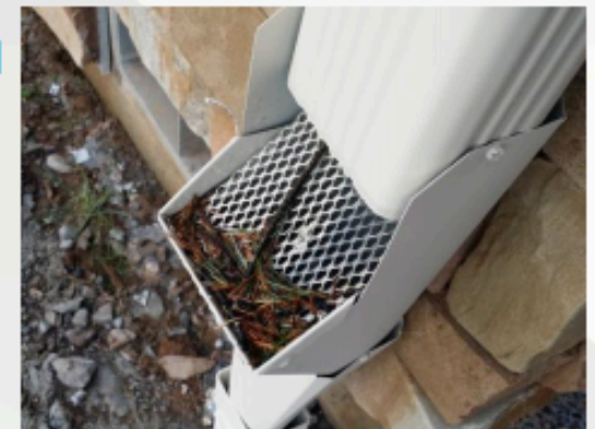
Right: Quail's standard gutter with cleanout
